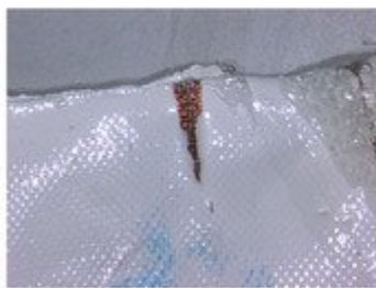
(c) Cracks in protective coating. (Reprinted from [71])
