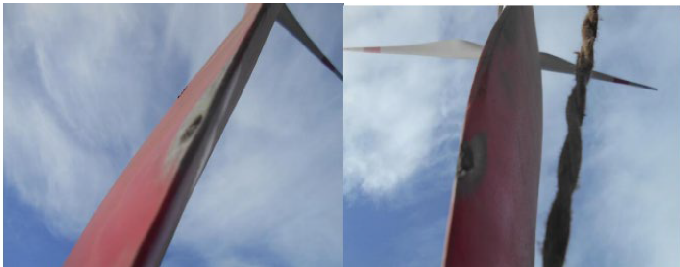
Figure 3. Holes in wind turbine blades caused by lightning strikes.
