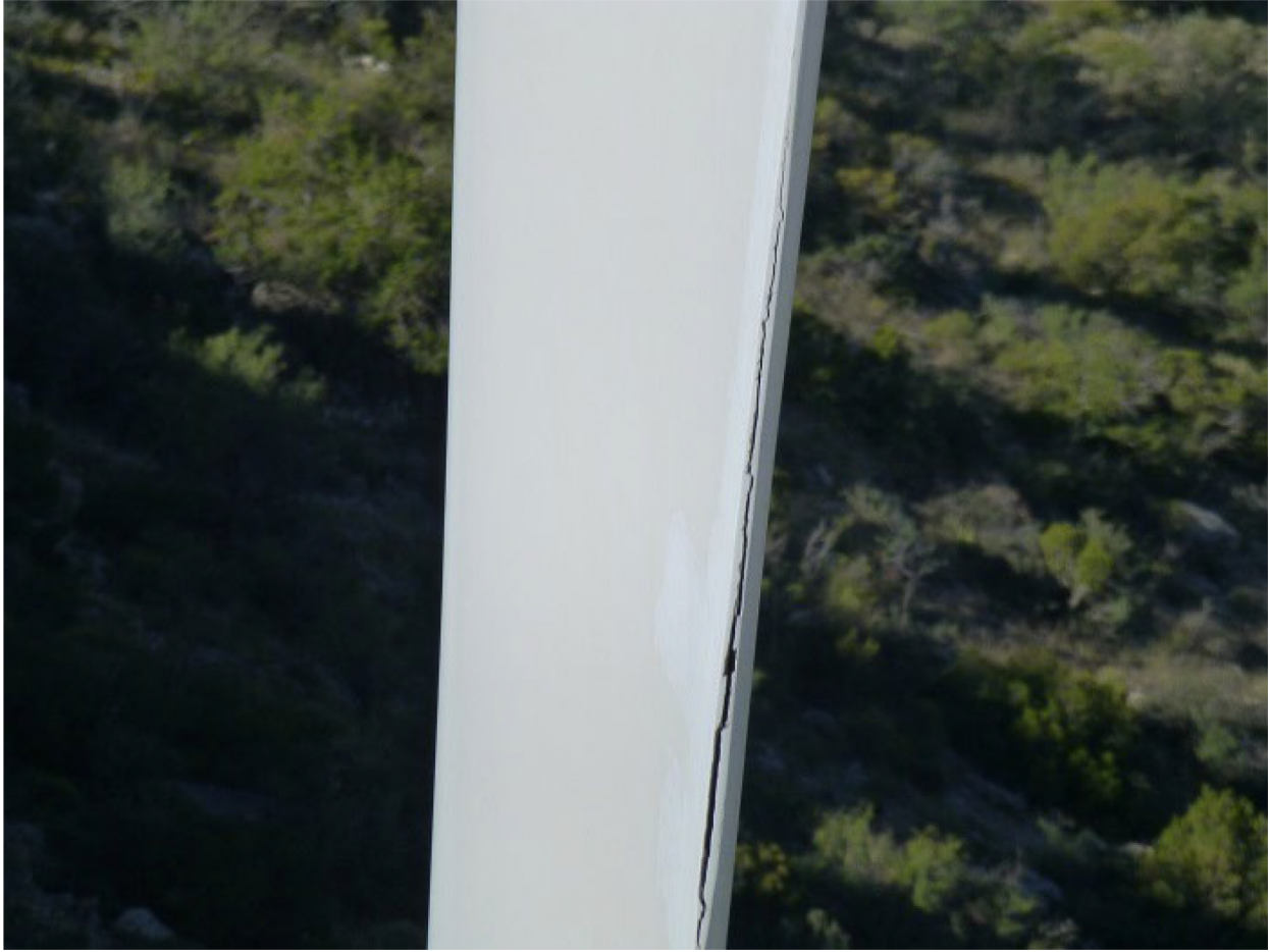
Figure 1. Longitudinal cracks found on the trailing edge of a wind turbine blade.
