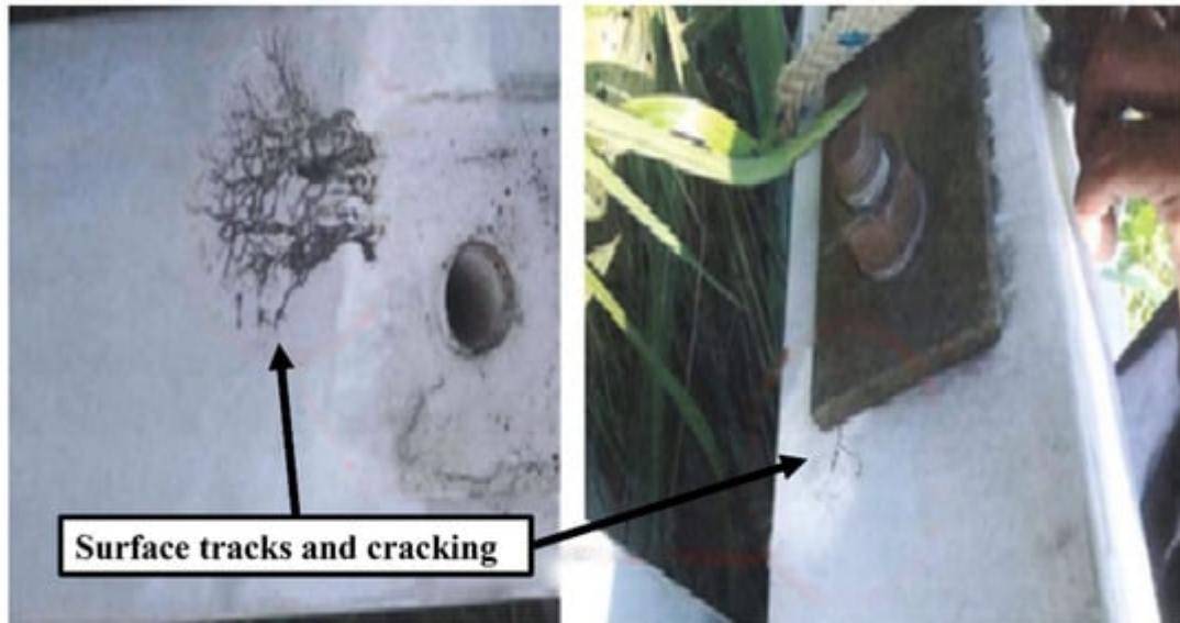
Figure 21. Surface tracking and cracks on the composite cross [60].
