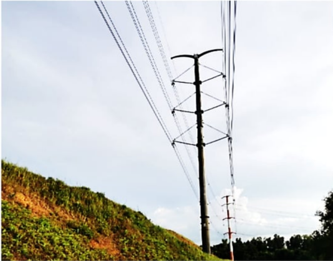
Figure 4. An example of TNB's compact composite tower line erected in Cyberjaya Selangor [12] .
