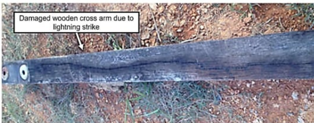
Figure 5. Failure of the wooden cross-arm due to lightning [14] .
