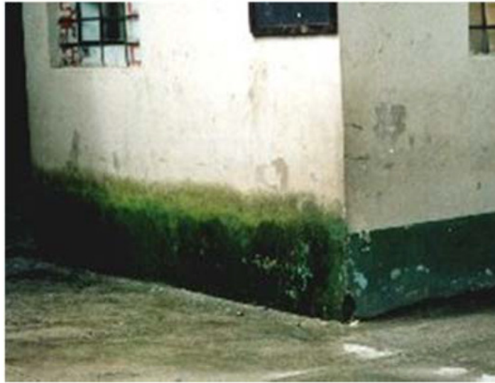
Figure 1. Heavy algal growth on the wet pediment of a building in Aguas Caliente, Peru.
