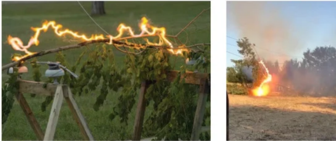
Figure 1. Vegetation-related faults and flashover in conductors [20].
