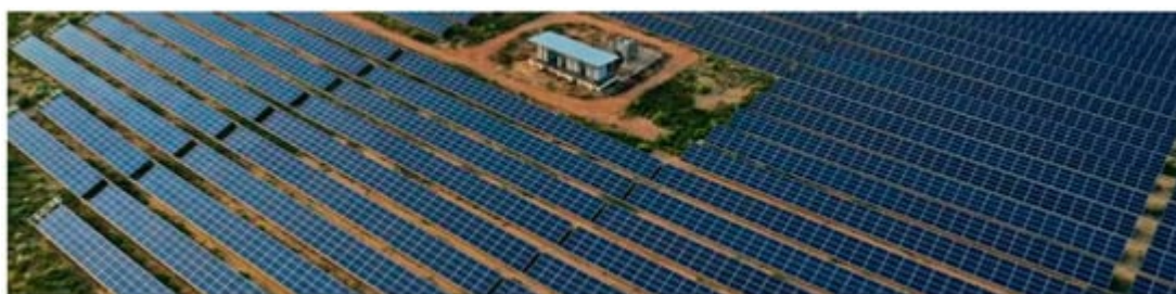
Figure 7. Bhadla solar park in India [16].
